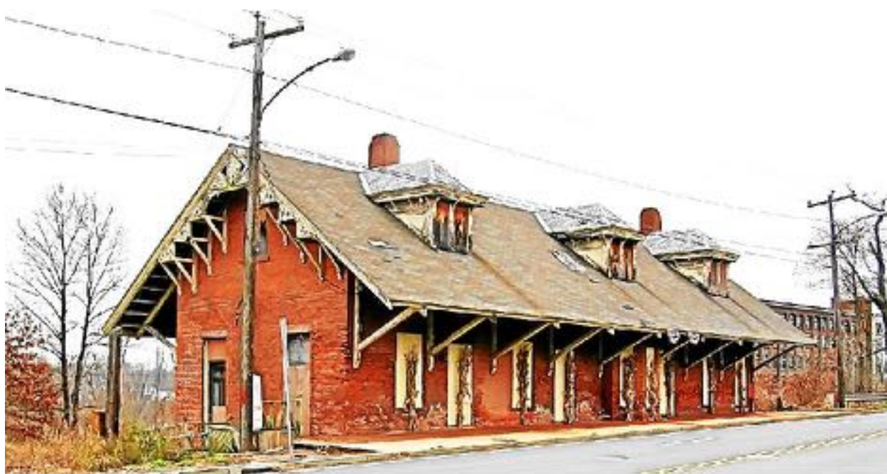
Passenger Station in deep decay ~ 2005
